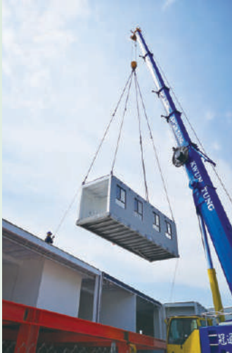
The O-PARK2 site office is built using the “Modular Integrated Construction” (MiC) method
